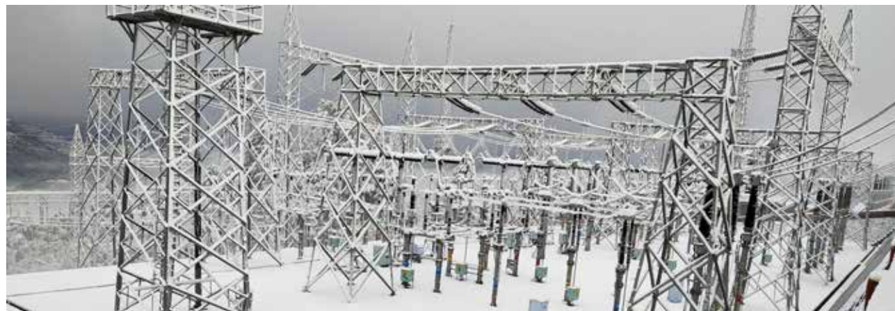
View of Pithoragarh Substation
